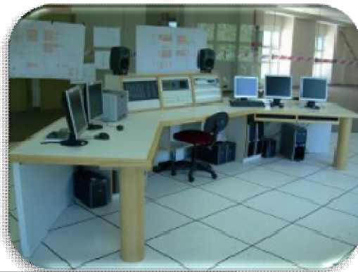
Master Control Room (MCR)
